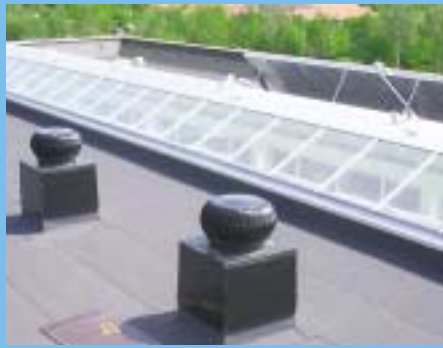
Wind driven roof mounted coils in Aabenraa Hospital
