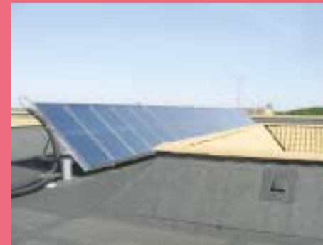
Solar collectors on the roof
