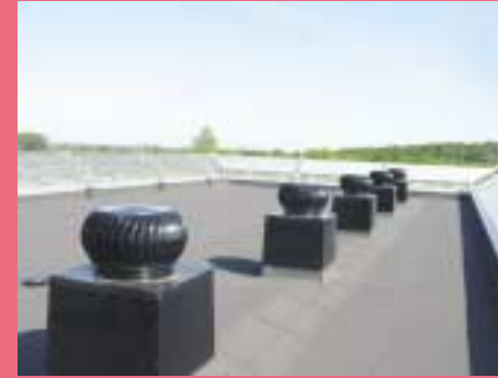
The wind cowls for natural ventilation
